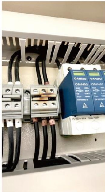
即時故障排除 Real-time Fault Resolution
